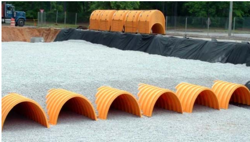
Fig.20 - StormTech Attenuation System
